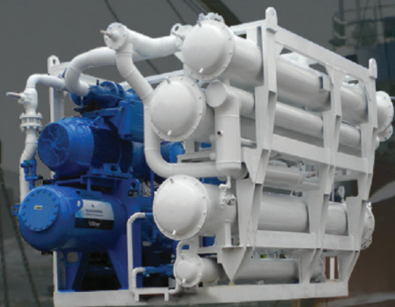
240 TR system with Ammonia
